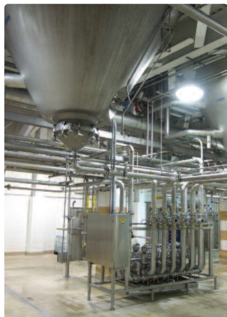
Plenty of room to work below these conicals at Shiner in Texas USA.
