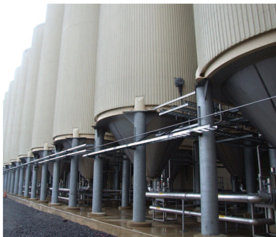
Even the vessel cones do not need to be enclosed. Frost protection is essential for a chilly winter in Virginia though – MillerCoors at Shenandoah, USA.
