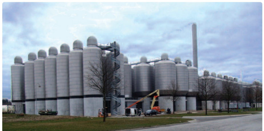
Putting finishing touches to the tank farm at Carlsberg, Fredericia in Denmark. 22 tanks were moved from the closed plant at Valby in Copenhagen, Denmark.
